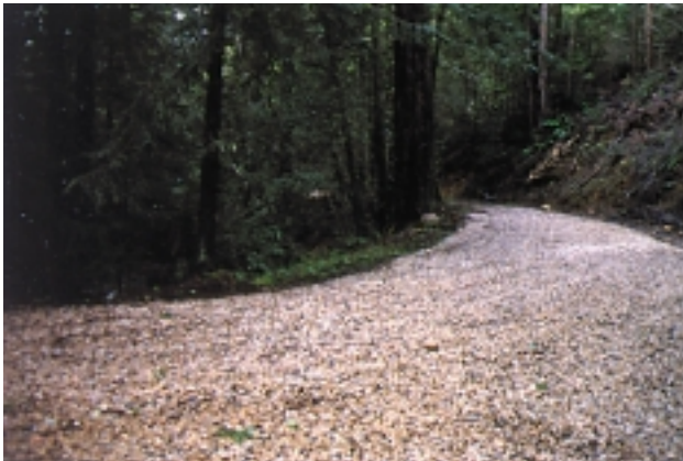
Figure 7. Rocked surface at crossing
