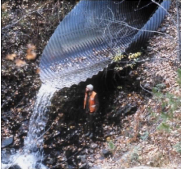
Figure 1. Fish can't get through here?
