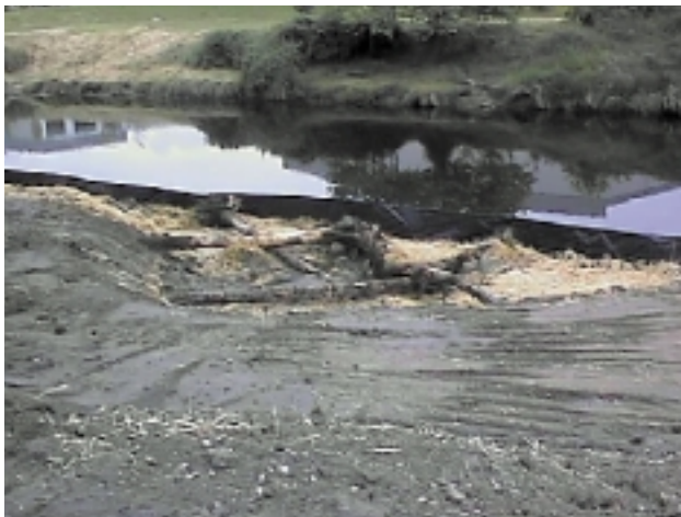
Figure 4. Silt fence along the Sammamish River
